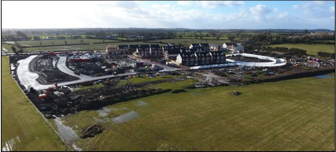
Figure 3: Recent aerial view of Phases 1A and 1B of The Willows under construction to the south of the SHD site
